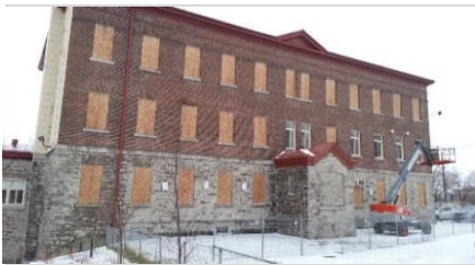
Ecole St. Edouard 2 Accublocs, total 6'850m 3 /h
